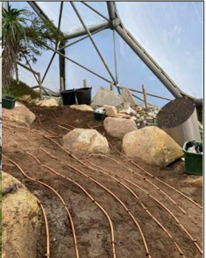
Laying out the irrigation lines before they get buried in the Mediterranean Biome.
